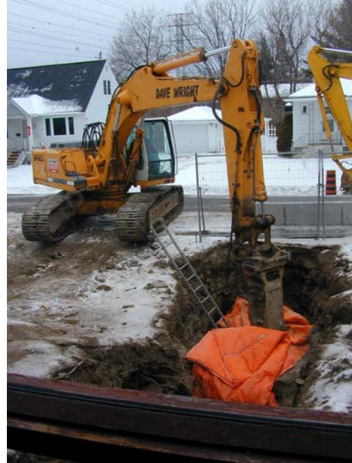
Ground vibrations due to construction equipment may damages foundations
